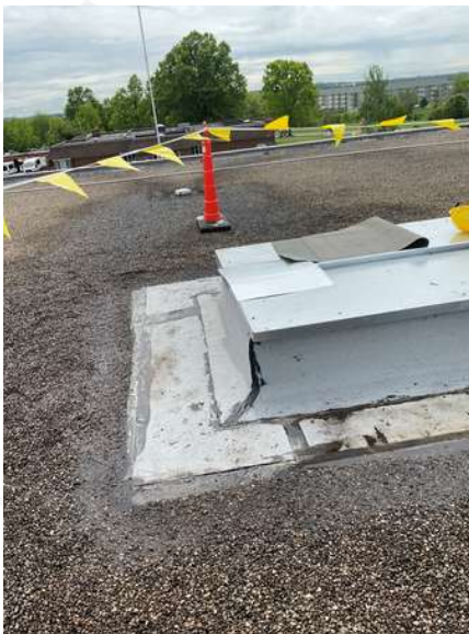
Roof Curb for RTU
