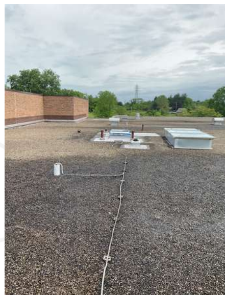
Roof supports for RTU
