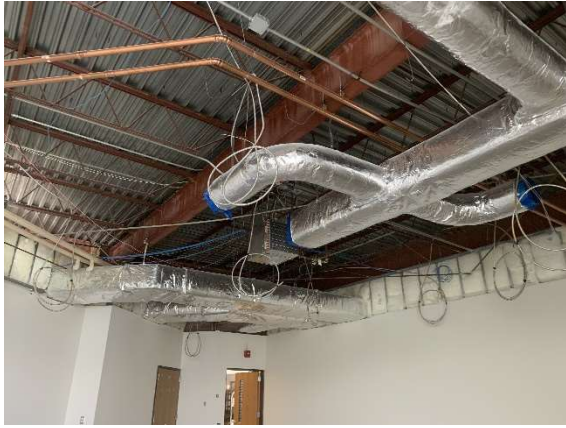
Ductwork – 80 Pod Classroom
