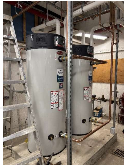
New Water Heaters – Mechanical Room
