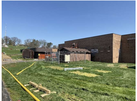
New Gas Service Line
